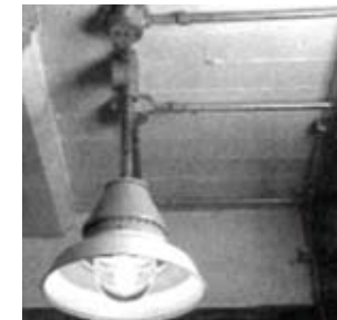
Typical Class 1 Div 1 conduit installation
