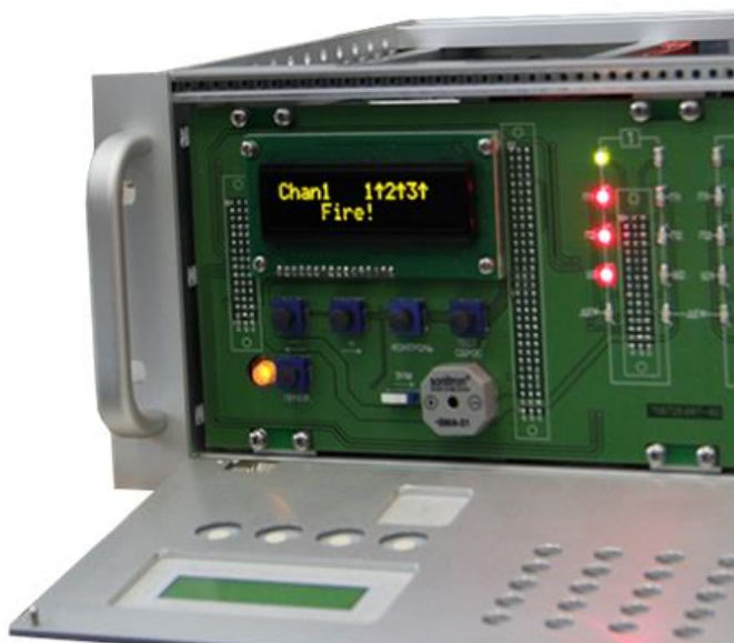
Fig. 3.1. Fire indication accompanied by audible alarm.
